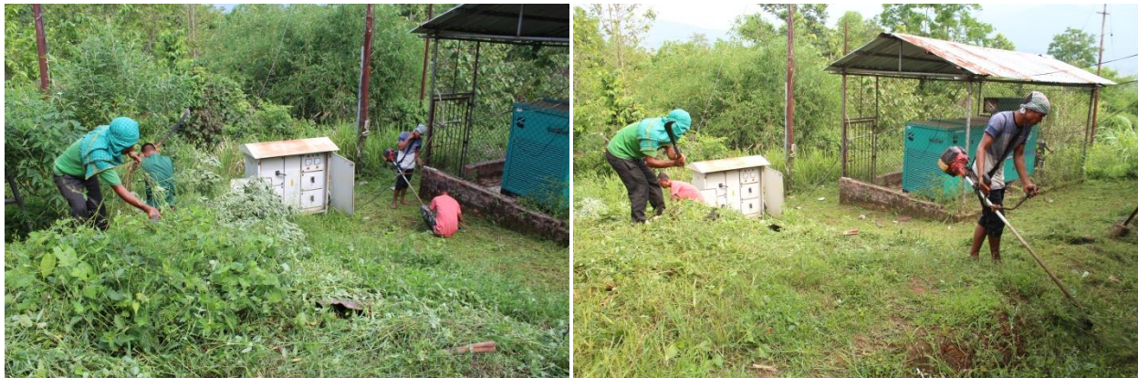
Cleaning of jungle around DG set
